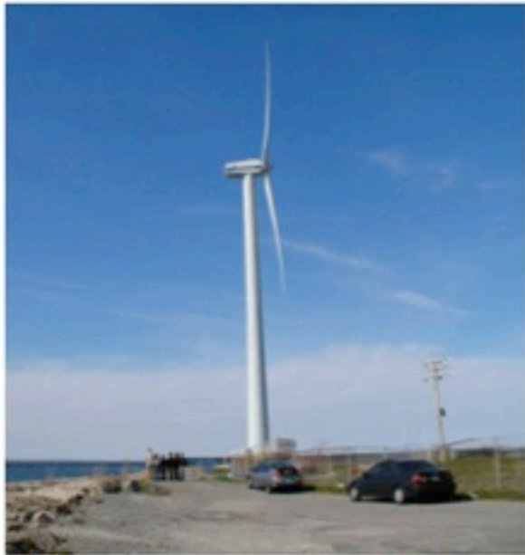
The Hull Muni generates wind power
