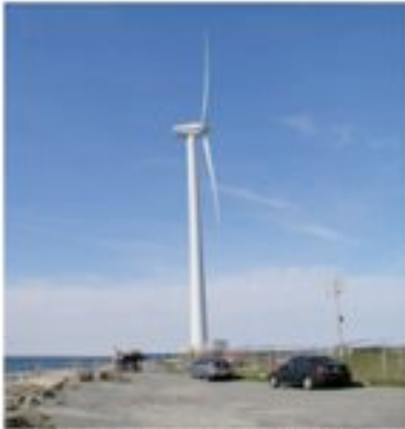
The Hull Muni generates wind power
